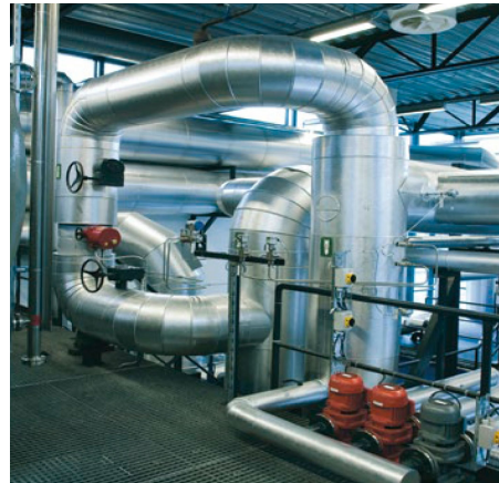
District heating production
