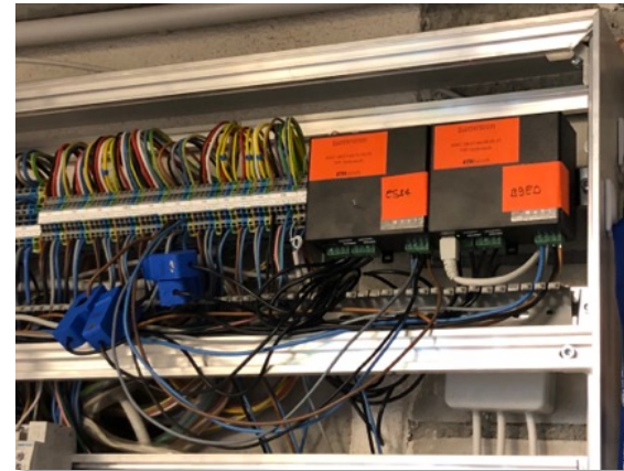
First installed devices (September 2018)
