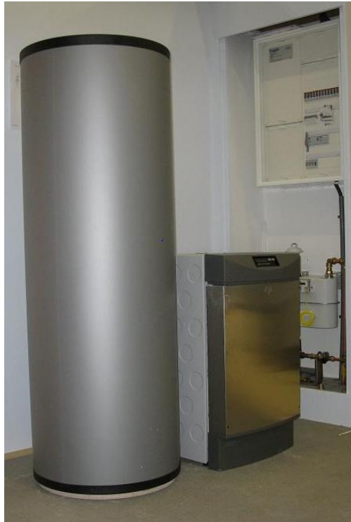
Figure A-3: Heating system with storage of tap water and heating water
