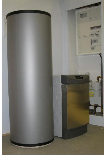
Figure A4 4. A storage tank along a micro-CHP
