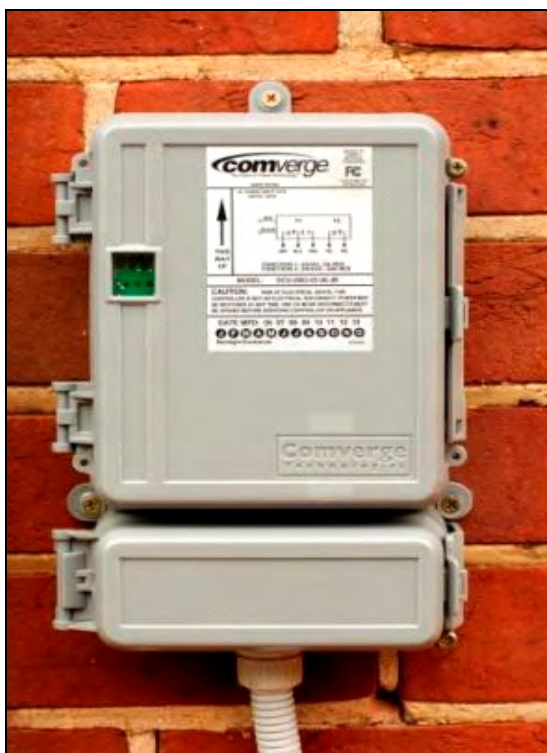
Figure 3. Comverge Load Control Unit Used in the ETSA Utilities Air Conditioner DLC Phase I Project
