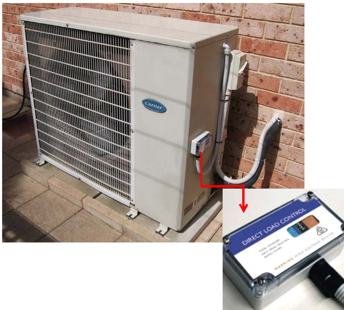
Figure 17. Saab Systems “Peak Breaker” Direct Load Control Device
