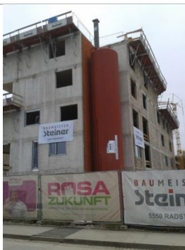
Figure 1: Smart building with 5 level high heat storage tank (source: Salzburg AG)
