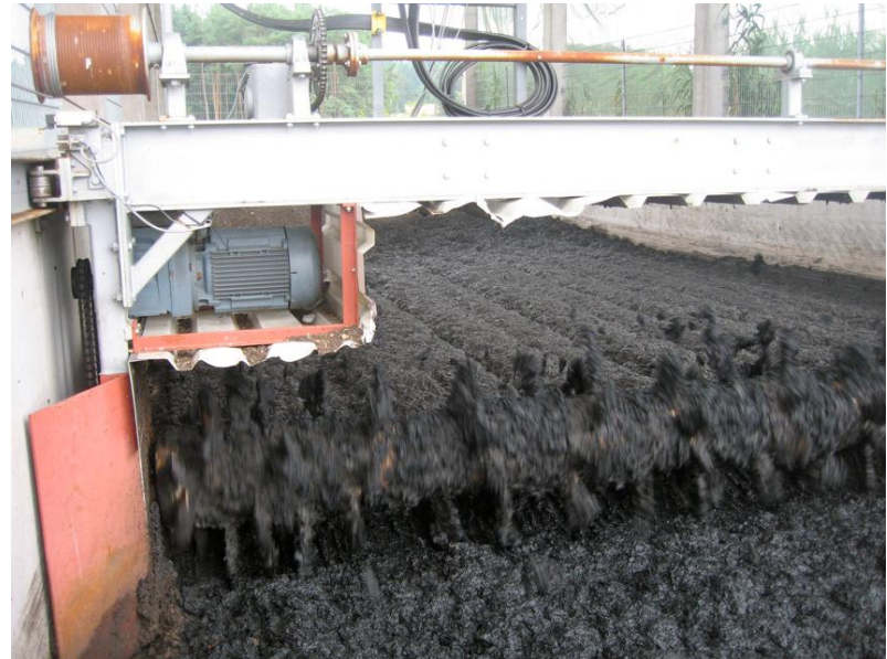
sludge turner, source: project GAVE
