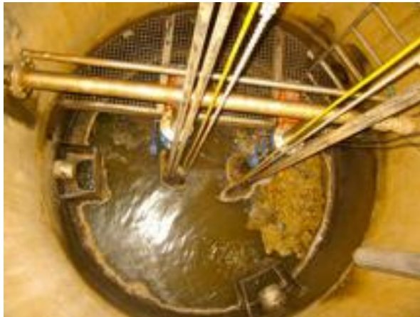
slurry pump, source: project GAVE
