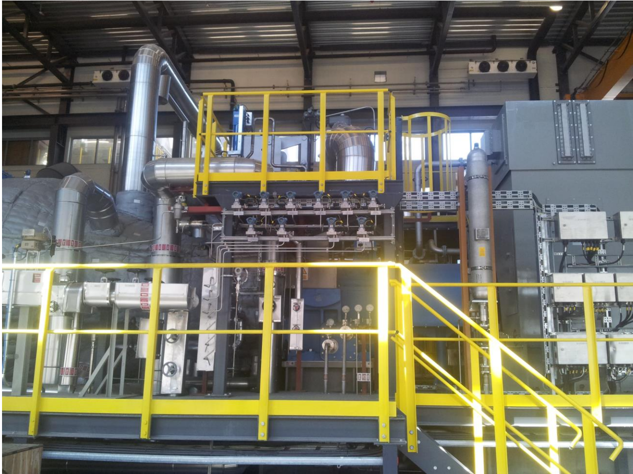
Inside the new heat recovery plant control room which is attached to the main production plant. Photo: Henrik Karlstrøm
